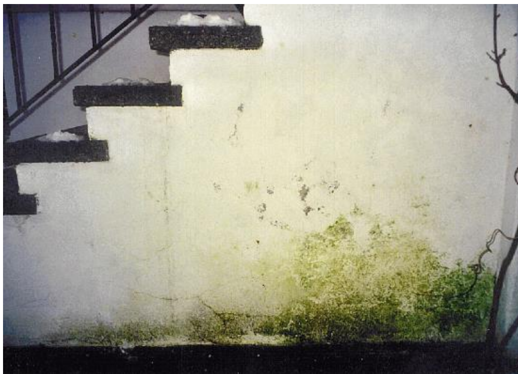
Figure 3. Fungal and Algal Growth on a Façade
