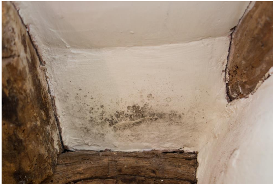
Figure 1. Mould Growth on a Painted Surface
