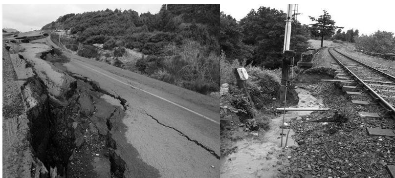
Figure 2.9. Foundation washout and collapse
