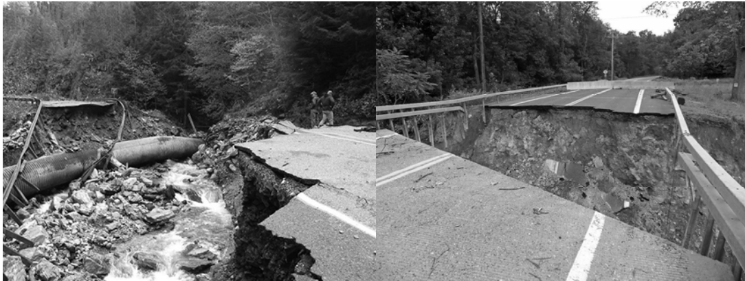
Figure 2.14. Road damage from culvert failure and washout
