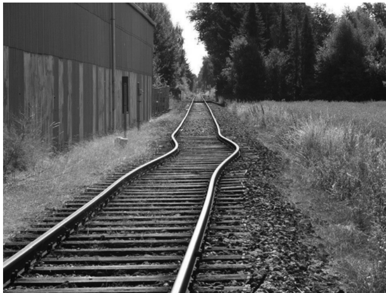
Figure 2.18. Heat-induced track buckling
