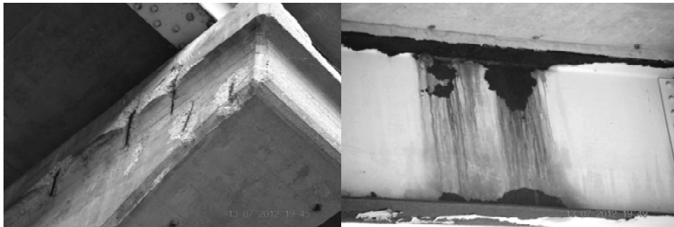
Figure 2.11. Steel and concrete bridge component corrosion
