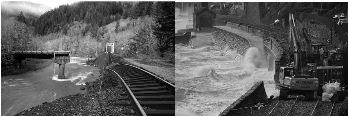
Figure 2.16. Impacts of storm-related embankment scour
